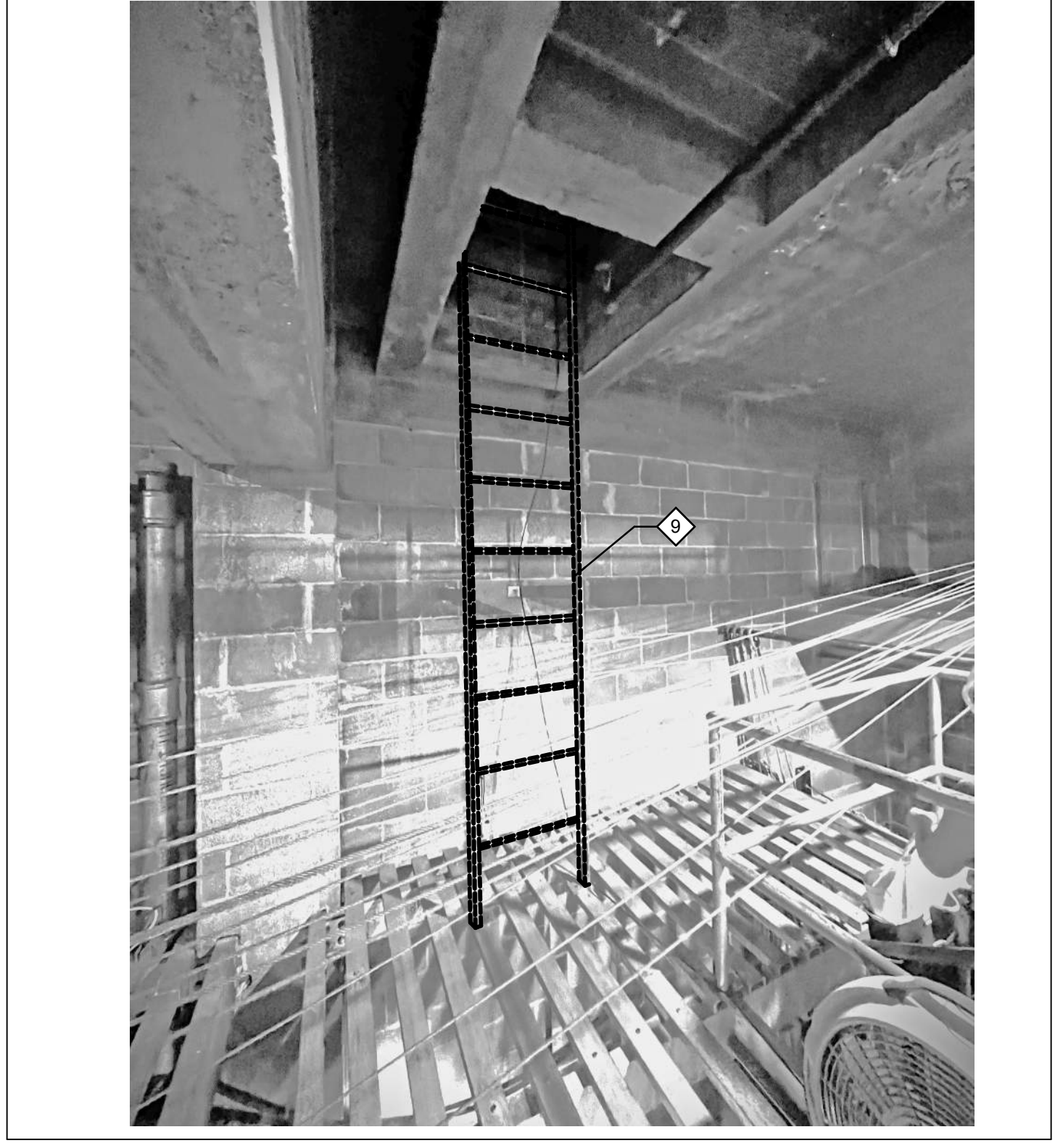
ROOF HATCH LADDER | B13
